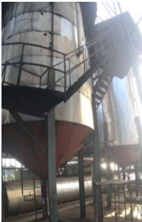
Vertical Claifier Tank
