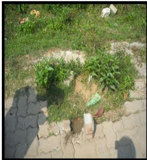
Gambar 2.5 : Paving block ditumbuhi rumput (Sumber : hand book on concrete block paving,2019 )
